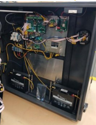
Sign Activated via SmartSign
