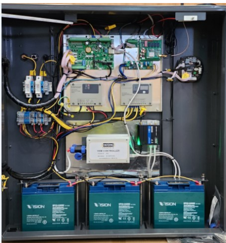
Sign Activated via SmartSign
