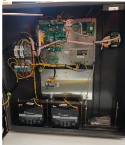
Sign Activated via Local Controller
