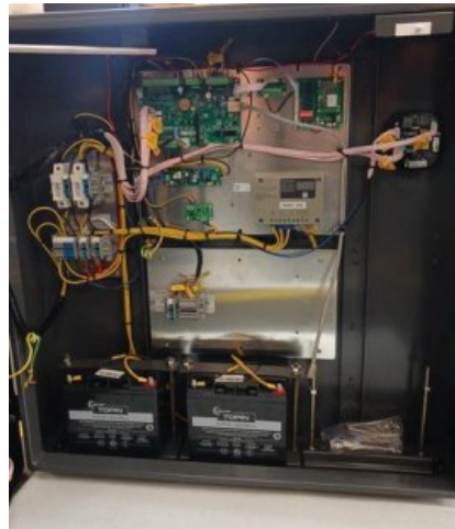
Sign Activated via Local Controller
